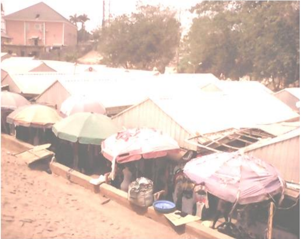
Plate IV: Open Stall Buildings in Garki Model Market with Inadequate Spaces between them (Source: Researchers' Field Work, 2018).
